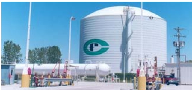
Fig. 7. “Atmospheric” refrigerated liquid anhydrous ammonia (NH 3 ) tank stores 190,000 MWh as 30,000 MT of NH 3 fuel. Total capital cost ~$ 15M; ~ $ 0.10 / kWh
