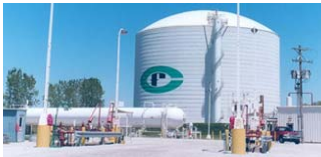
Figure 10. Liquid anhydrous ammonia ( \text{NH}_3 ) storage tanks. Foreground: 10 bar, ~ 100 ton, carbon steel "bullet" tank, appropriate for Alaska village storage. Rear: 1 atm, ~ 30,000 ton, -33 C refrigerated, double-wall steel tank, appropriate for large Alaska communities and for firming seasonal hydro plants.
