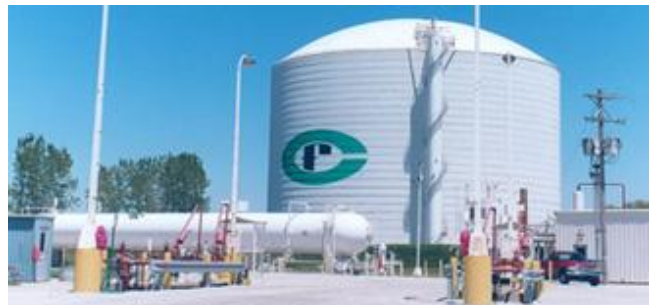
Fig. 7. “Atmospheric” refrigerated liquid anhydrous ammonia (NH 3 ) tank stores 190,000 MWh as 30,000 MT of NH 3 fuel. Total capital cost ~$ 15M; ~ $ 0.10 / kWh
