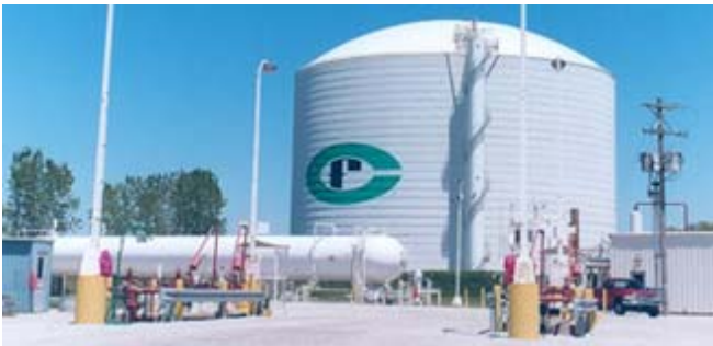
Figure 10. Liquid anhydrous ammonia (NH 3 ) storage tanks. Foreground: 10 bar, ~ 100 ton, carbon steel “bullet” tank, appropriate for Alaska village storage. Rear: 1 atm, ~ 30,000 ton, -33 C refrigerated, double-wall steel tank, appropriate for large Alaska communities and for firming seasonal hydro plants.
