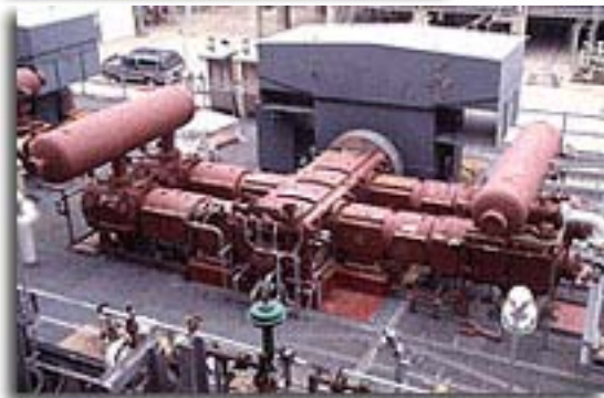
5500 horsepower HHE-VL hydrogen make-up compressor.
